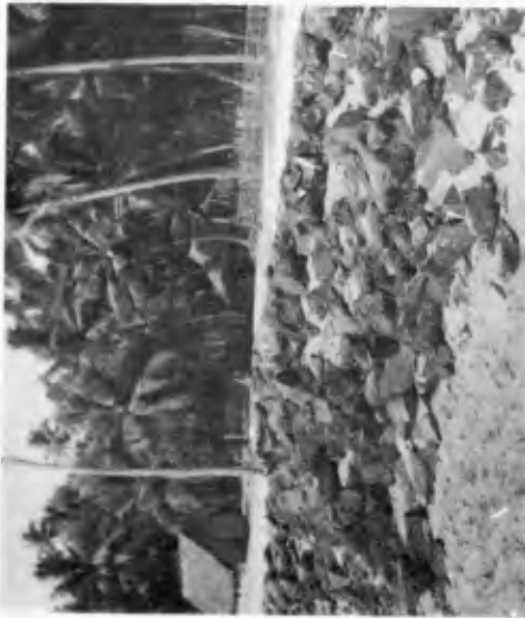
Fig. 4. Damage to sea wall constructed with bituminous grouting.
